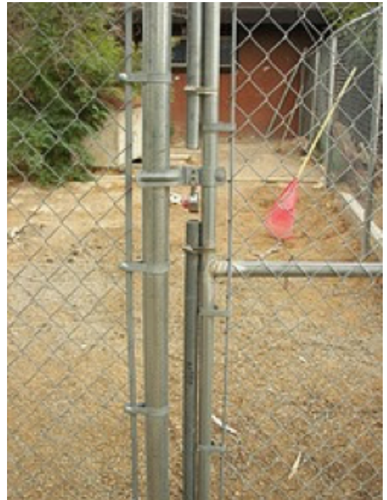
Gap fixed by clamping on conduit
